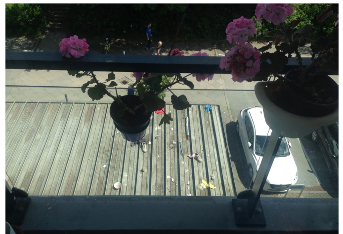
Figure 67 Example of waste on canopy roofs. Figure 67 was not part of the original published paper.
