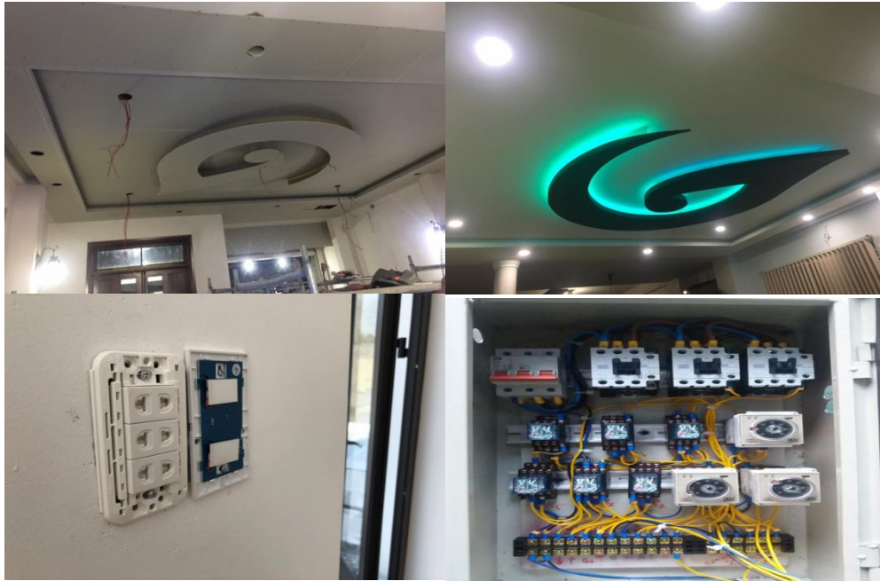
Figure 4. An example of smart home installation
